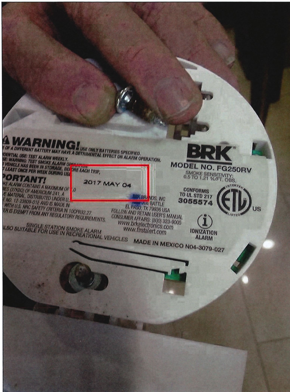
Smoke Detector Data Plate
